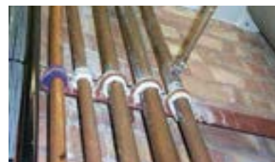
Figure 29 Chrysotile cloth on pipes
