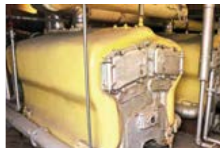
Figure 13 Amosite lagged boiler with hard plastic coating
