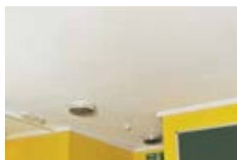
Figure 36 Asbestos textured coating on ceiling
