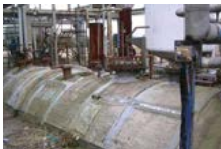
Figure 12 Lagging on large petrochemical vessel
