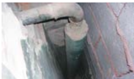
Figure 9 Lagged pipe in wall cavity
