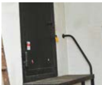
Figure 45 'Durasteel' composite steel and asbestos fire door
