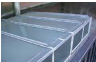
Figure 31 Chrysotile string on skylights
