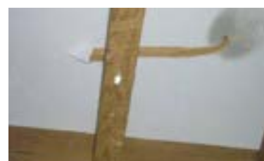
Figure 25 Chrysotile paper on strawboard ceiling panels
