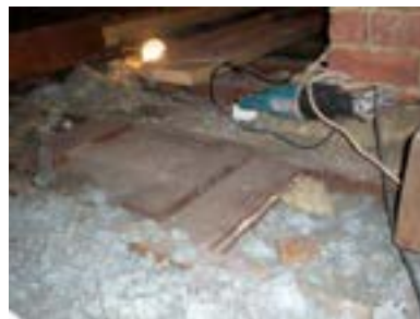
Figure 6 Loose asbestos used as loft insulation
