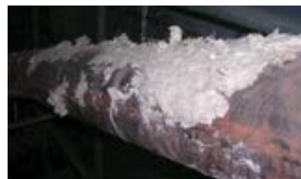
Figure 11 Amosite lagging in very poor condition on steam pipe
