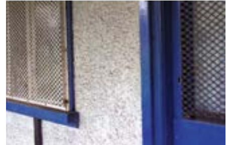
Figure 33 Chrysotile pebble-dash exterior wall coating
