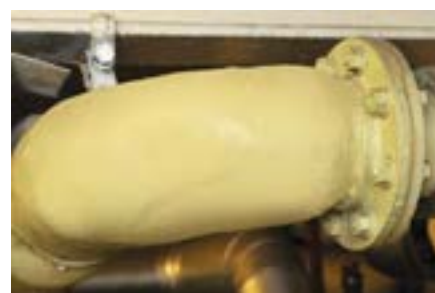
Figure 10 Pipe insulation with coating
