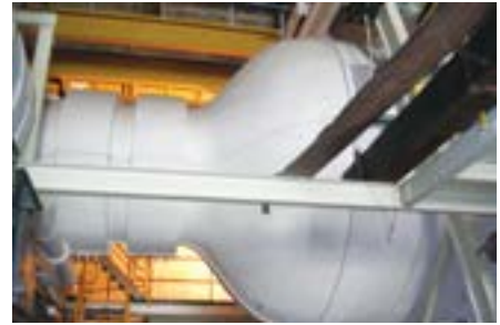
Figure 51 Vessel clad in amosite insulation
