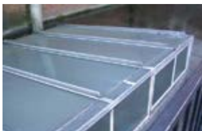
Figure 31 Chrysotile string on skylights
