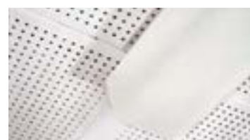
Figure 17 AIB ceiling tiles
