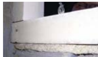
Figure 27 Amosite asbestos rope packing on riser door frame
