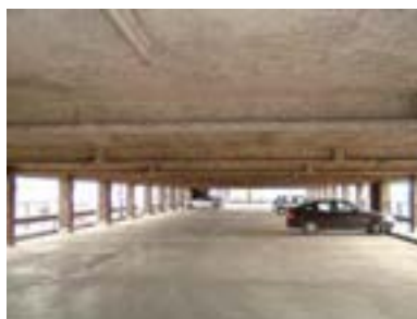
Figure 7 Sprayed limpet on car park roof
