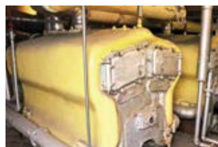
Figure 13 Amosite lagged boiler with hard plastic coating
