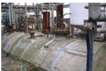
Figure 12 Lagging on large petrochemical vessel
