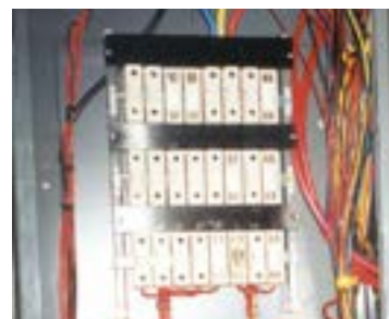
Figure 46 Asbestos tape flash guards in a fuse box
