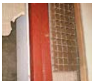
Figure 21 AIB column fire protection in CLASP building
