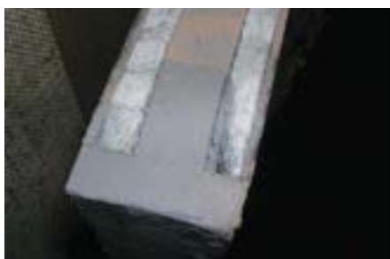
Figure 14 Asbestos panels inside fire door
