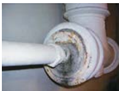
Figure 30 Amosite and chrysotile packing on waste pipes
