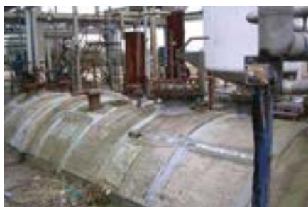
Figure 12 Lagging on large petrochemical vessel
