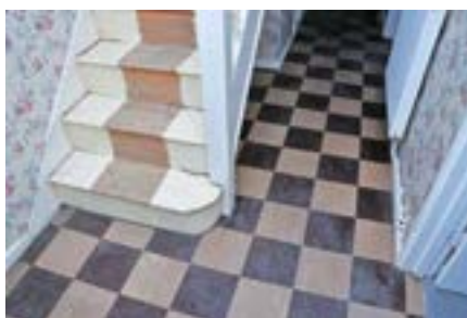
Figure 39 Asbestos-containing vinyl floor tiles
