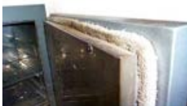
Figure 26 Asbestos rope seal on drying oven
