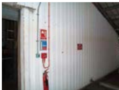
Figure 38 Chrysotile/bitumen coating under metal cladding
