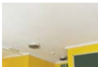
Figure 36 Asbestos textured coating on ceiling
