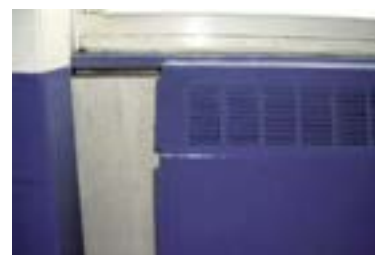
Figure 19 AIB behind school radiator unit
