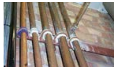
Figure 29 Chrysotile cloth on pipes
