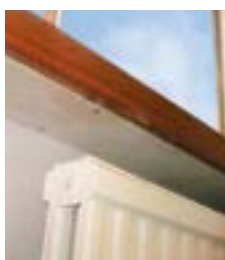
Figure 20 AIB panel between radiator and window
