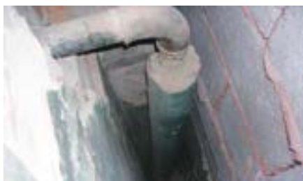
Figure 9 Lagged pipe in wall cavity
