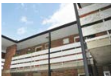
Figure 18 AIB exterior panel on open walkway
