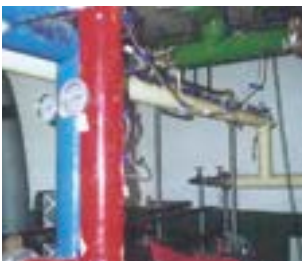
Figure 7.9 Good practice: Wet injection on pipework
