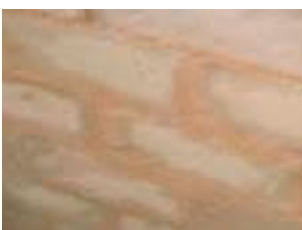
Figure 7.26 Remnants of asbestos on breeze blocks
