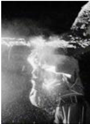
Figure 7.1 Uncontrolled dry stripping
