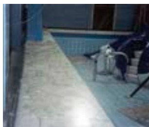
Figure 1.7 Uncontrolled removal of asbestos
