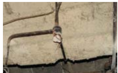
Figure 3 Sprayed asbestos insulation: work with this material requires a licence
