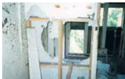
Figure 7 Asbestos insulating board wall panels badly damaged
