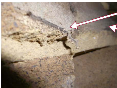
Figure A5.9 Remnants of asbestos on materials
