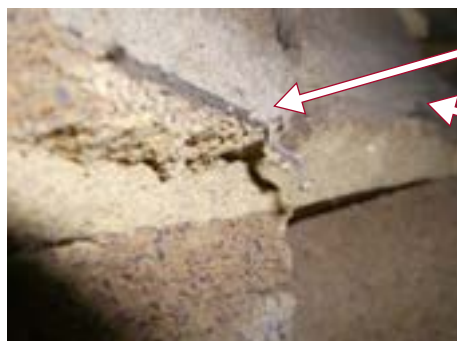
Figure A5.9 Remnants of asbestos on materials
